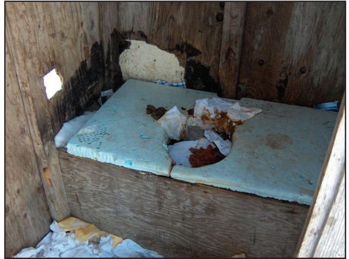
Photo of an overflowing outhouse in Pikangikum, part of the Inspection Report on the Pikangikum Water and Sewage Systems, Northwestern Health Unit, September 2006.
